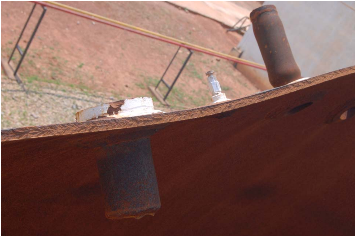
Photo 4: Swelling of stubs seen. The edge shows the thick brittle fracture.
