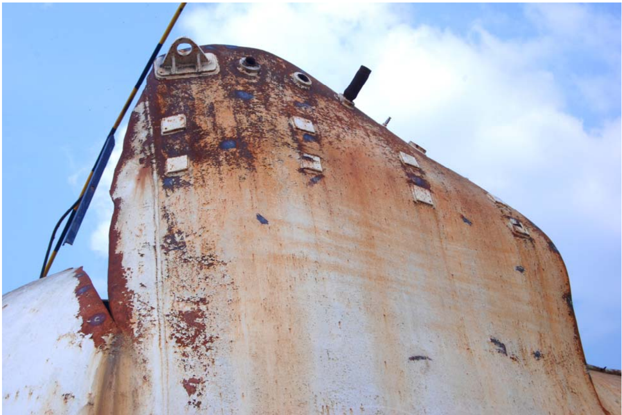
Photo 8: Failure seemed to have started at lifting lug zone and travelled on either side. The edge of failed section is thick. Hence this is a brittle fracture. The vessel must have turned brittle in service.
