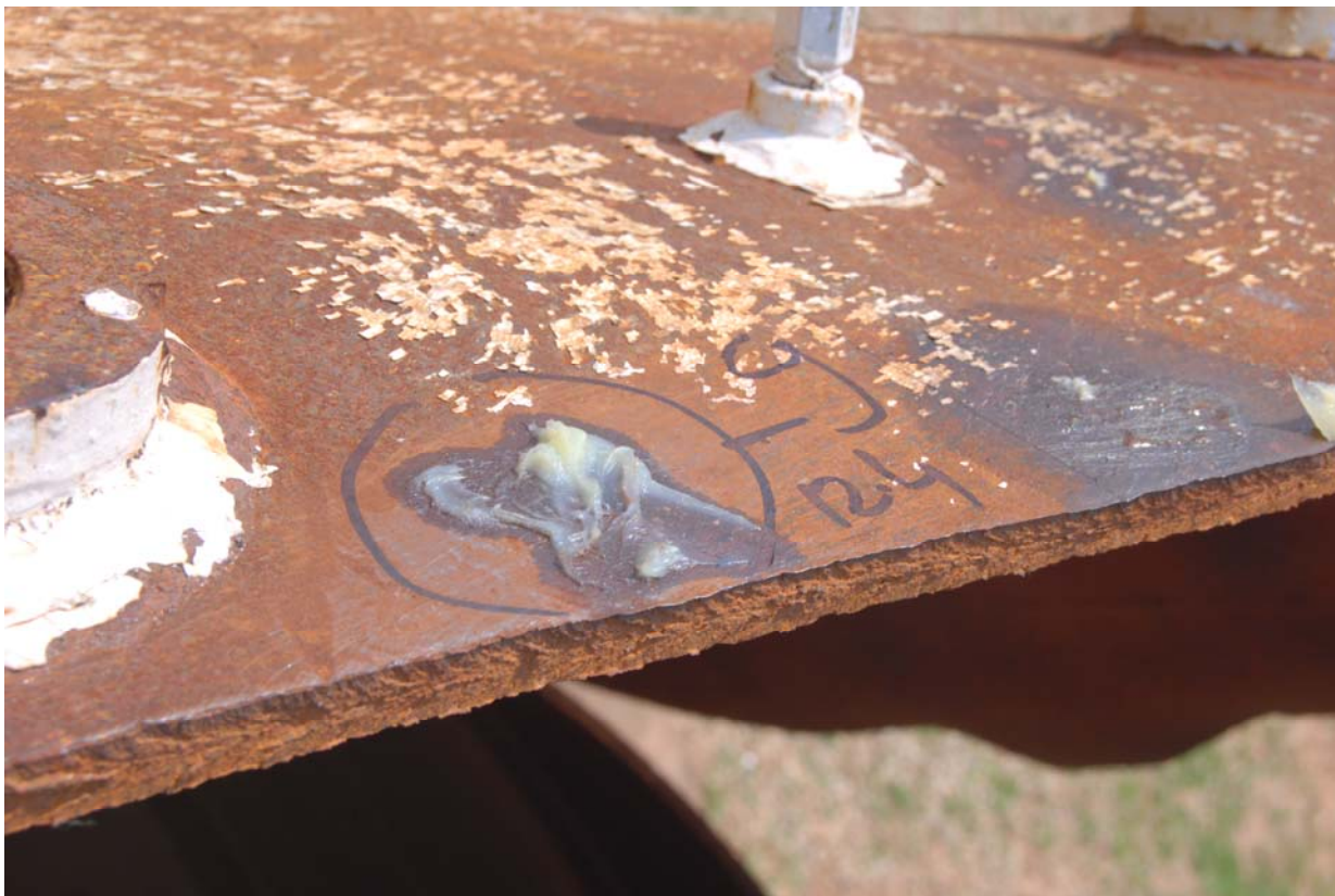
Photo 3: Along the failed edge no lamellar kind of defect is seen. No thinning is seen. This is a brittle failure. A section of plate from other place should be tested for impact test.
